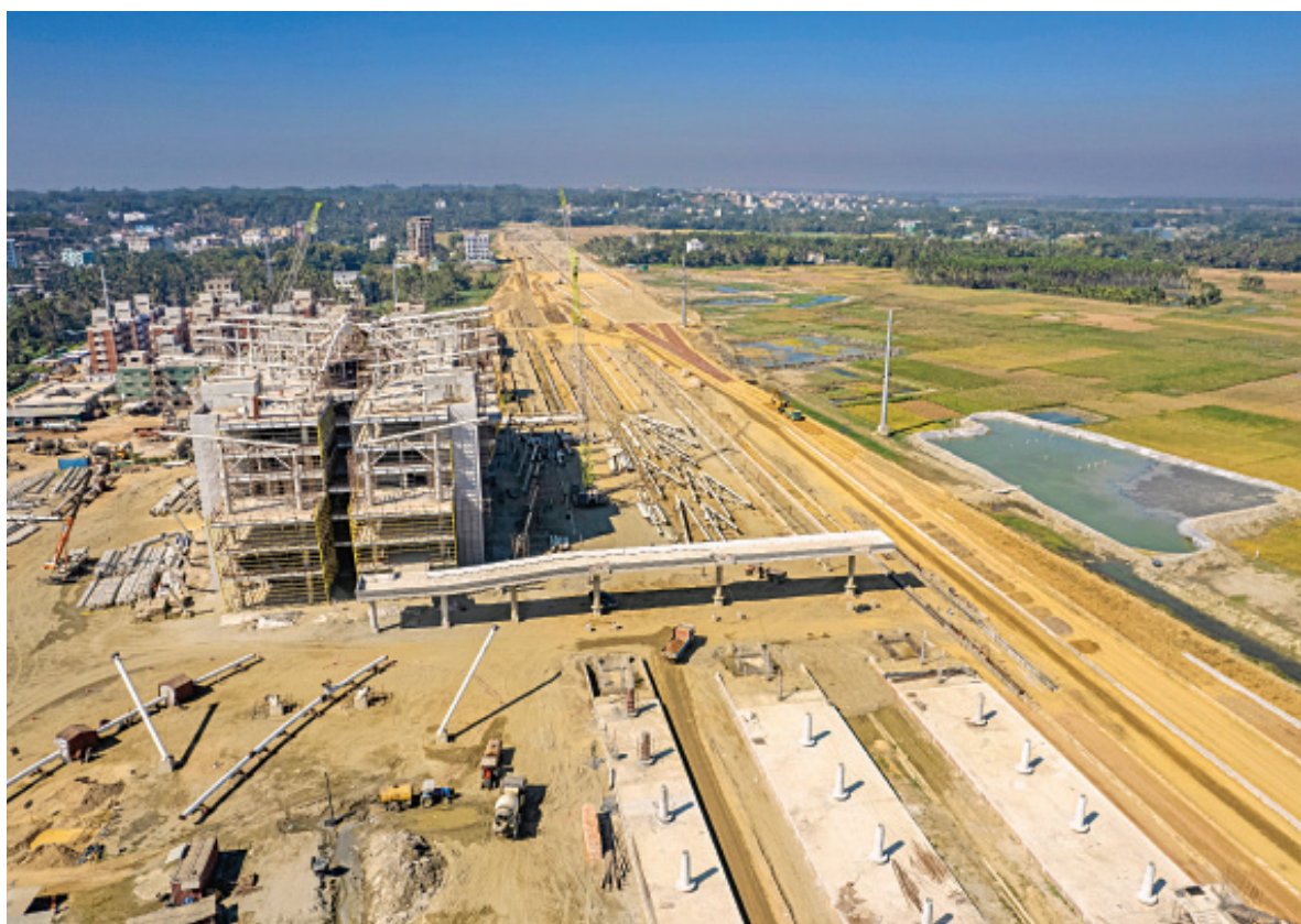
The construction of an iconic railway station in Ramu upazila of Cox's Bazar has been going on in full swing. Once built, the oyster-shaped station on 29 acres of land will connect the district with Chattogram and the rest of the country. The photo was taken in Ramu's Chandeparra area recently. PHOTO: RASHED SHUMON
