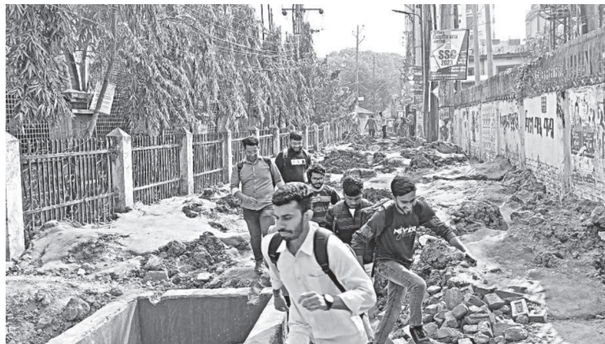
Students and pedestrians in general have been left to suffer for seven months due to unfinished roadwork beside Mymensingh's Alexander castle. This is a busy road as three educational institutions, a teacher's training institute and several government offices are located nearby. The photo was taken recently. PHOTO: STAR
