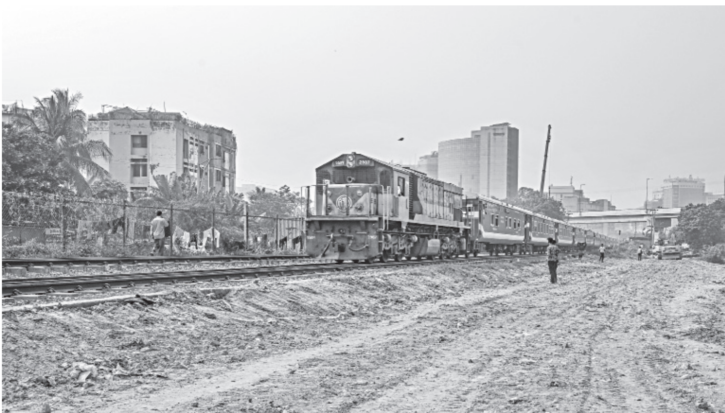
Workers are levelling the ground by the rail track in Tejgaon area for the construction work of the elevated expressway. This photo was taken yesterday.
