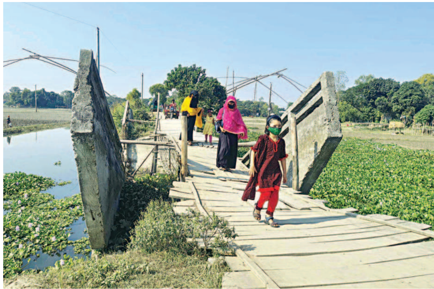
People crossing a damaged bridge over a water body at Karmakarpara in Tangail's Basail upazila. Vehicular movement remains suspended on the Hatkhola-Kanchanpur-Paschimpara road since the bridge was affected by floods in 2021, causing locals to suffer. The photo was taken recently.
