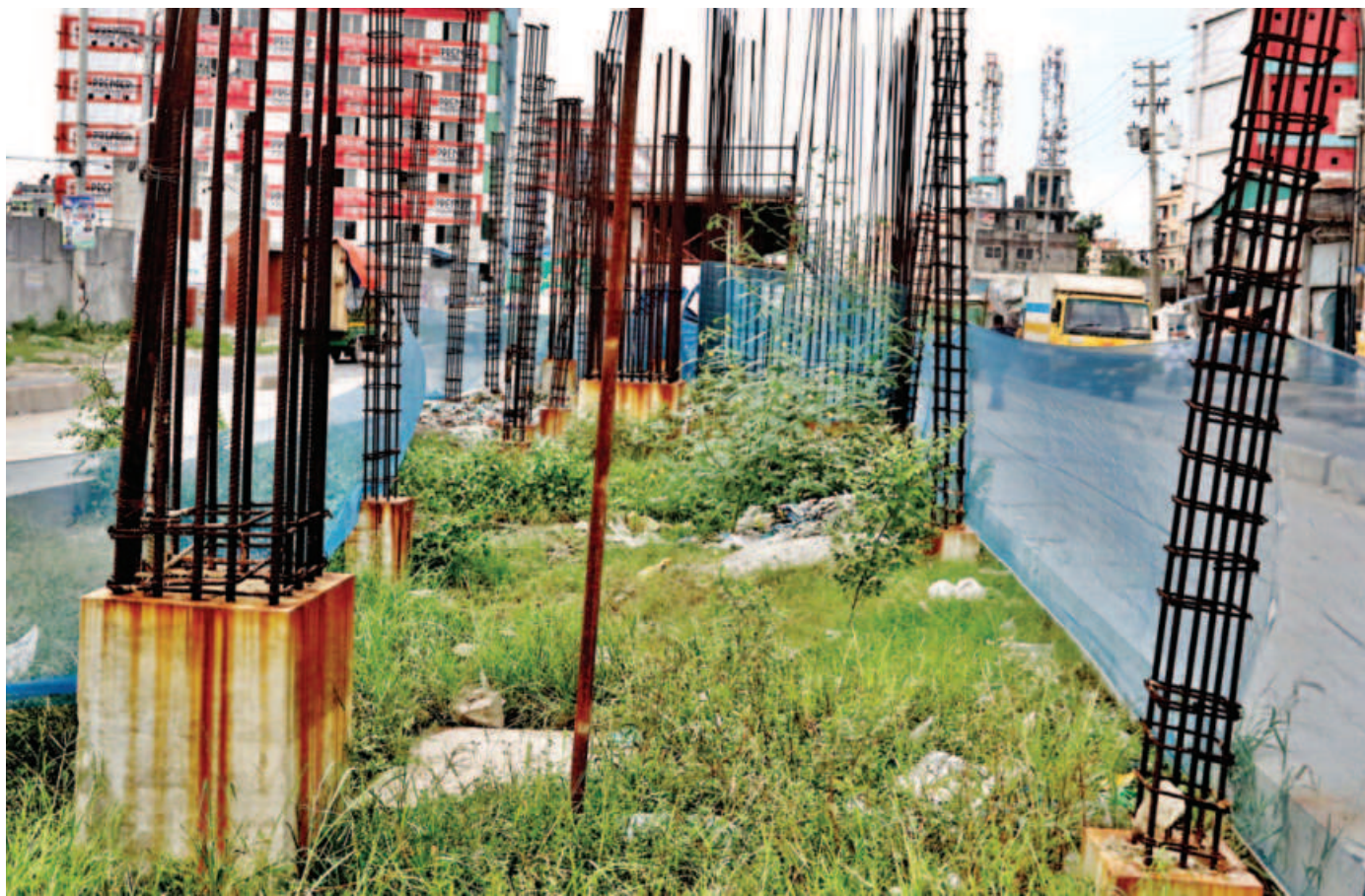
Unfinished pillars of Bus Rapid Transit (BRT) project have been left like this for months in Basan area of Gazipur. The BRT project was supposed to be completed in 2016. Its current deadline expires next month. The photo was taken recently. PHOTO: ANISUR RAHMAN
