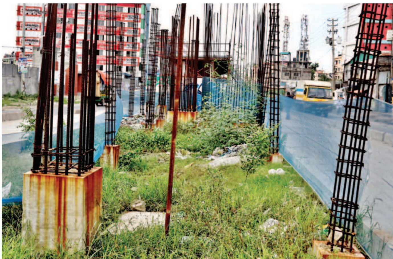
Unfinished pillars of Bus Rapid Transit (BRT) project have been left like this for months in Basan area of Gazipur. The BRT project was supposed to be completed in 2016. Its current deadline expires next month. The photo was taken recently.
