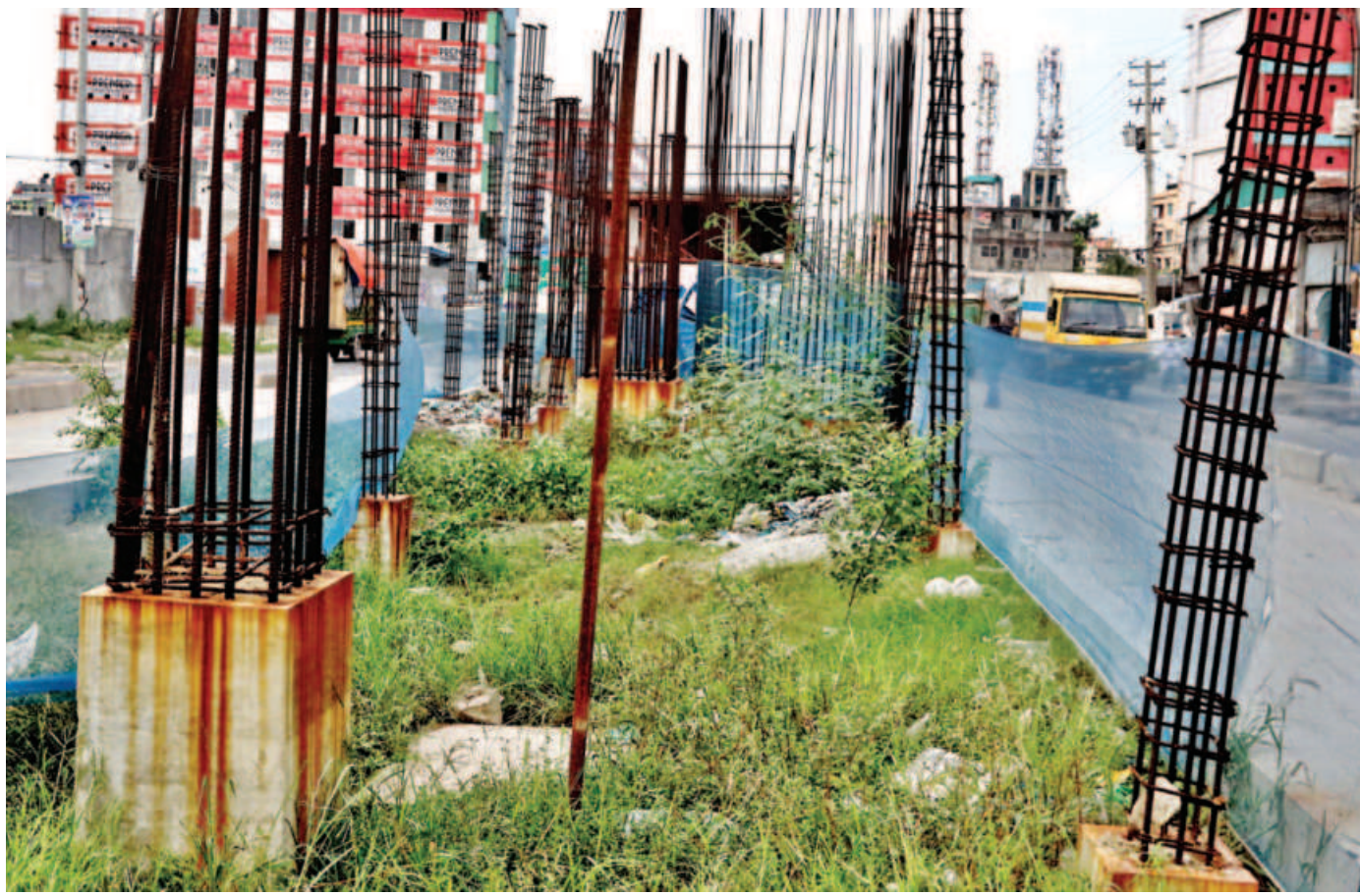
Unfinished pillars of Bus Rapid Transit (BRT) project have been left like this for months in Basan area of Gazipur. The BRT project was supposed to be completed in 2016. Its current deadline expires next month. The photo was taken recently. PHOTO: ANISUR RAHMAN
