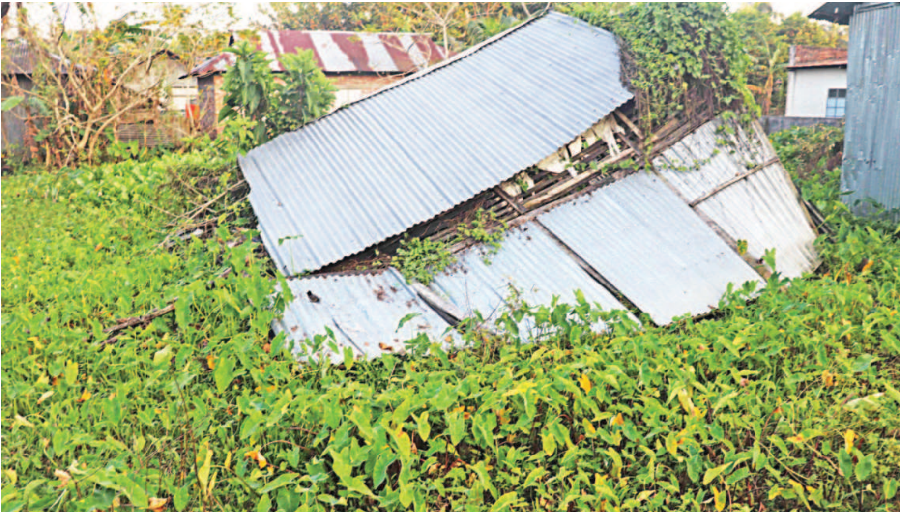
A collapsed shed is seen at an abandoned plot of the BSCIC industrial estate in Nesarabad upazila of Pirojpur. Many entrepreneurs who were allotted plots in the area are either renting them out to others or leaving them vacant considering the poor facilities present.
