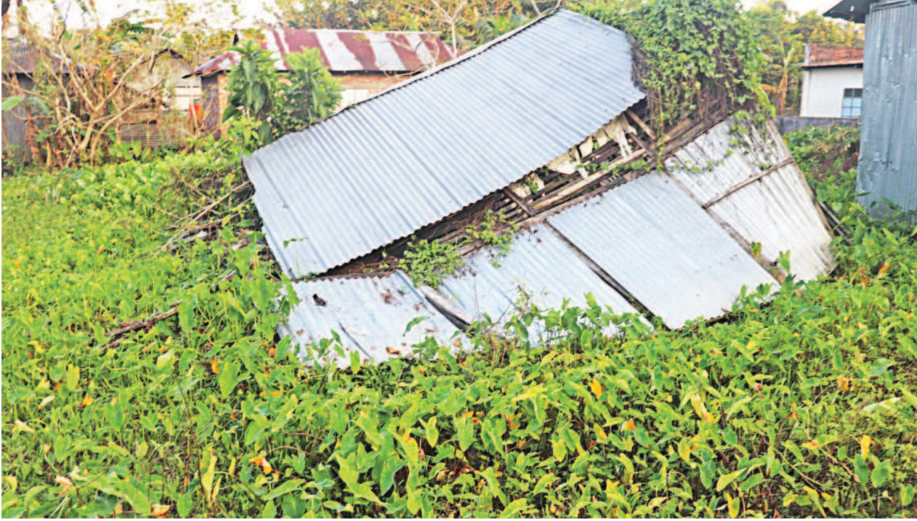
A collapsed shed is seen at an abandoned plot of the BSCIC industrial estate in Nesarabad upazila of Pirojpur. Many entrepreneurs who were allotted plots in the area are either renting them out to others or leaving them vacant considering the poor facilities present.
