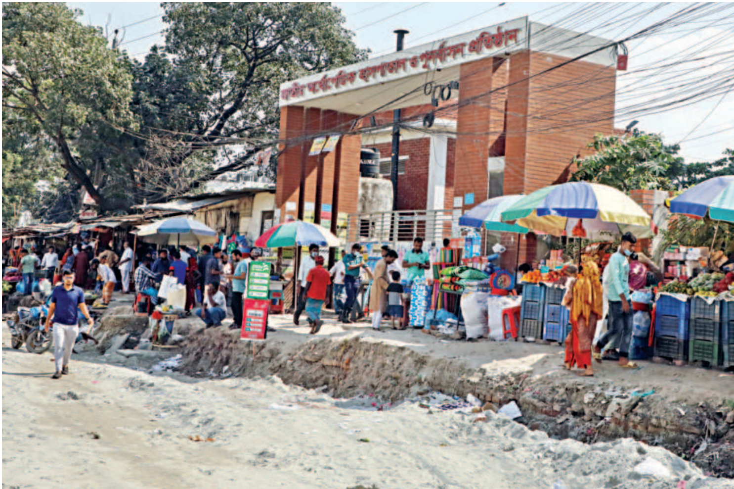
For months now, patients, their attendees and civilians have not been able to move freely on the road in front of National Institute of Traumatology and Orthopaedic Rehabilitation, as authorities have dug up a large section for development work. On top of that, vendors have also set up shop on the footpath, further restricting movement. This photo was taken recently.
