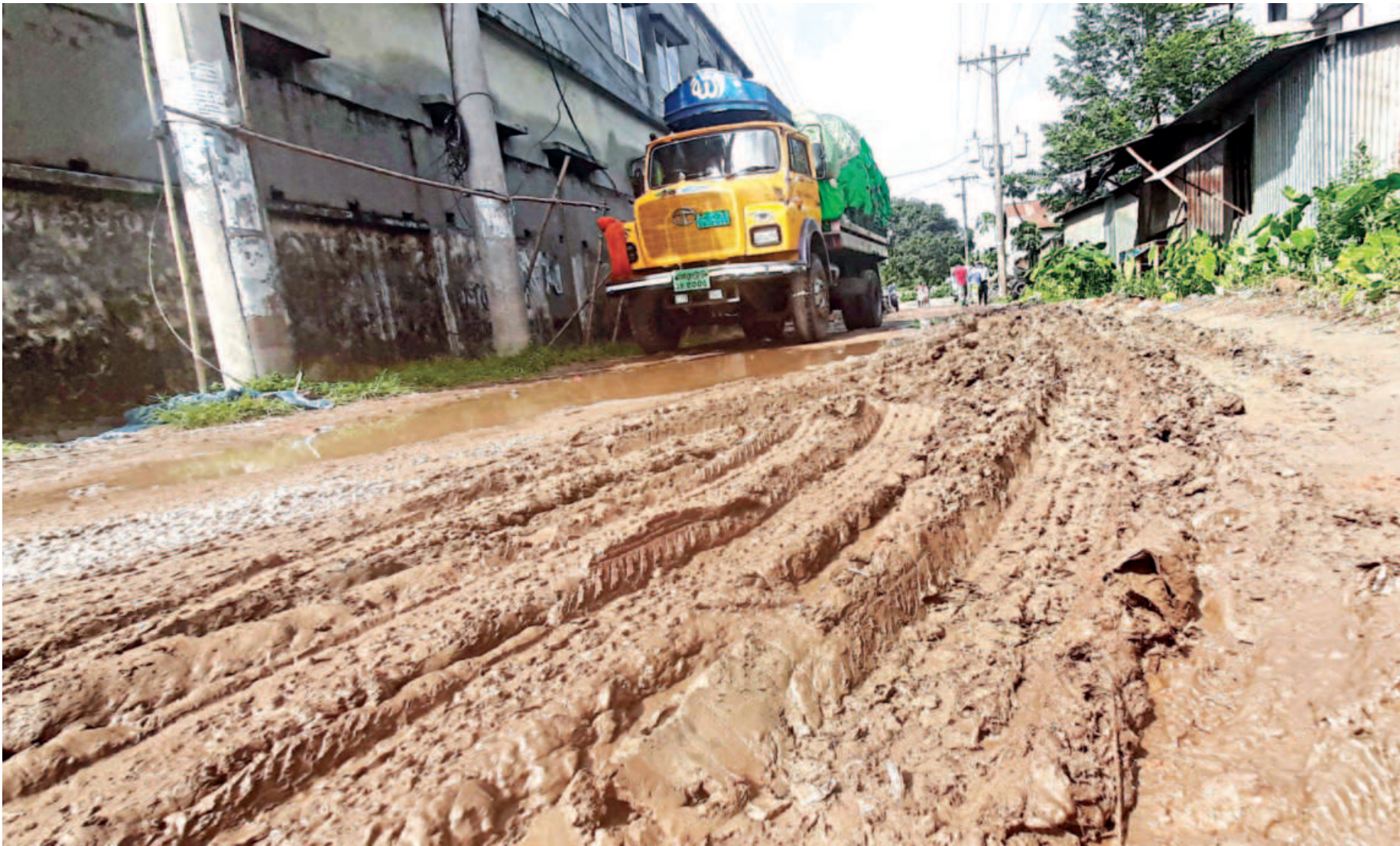
Trucks and other vehicles moving through the BSCIC industrial estate in Tangail leave deep gashes in their wake as the roads have become a slush of mud and water due to the poor drainage system. Meanwhile, an illegal kitchen market at the estate grants just about anyone access to the factory areas.
