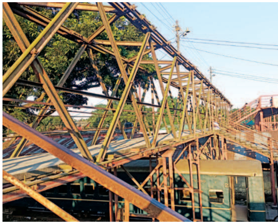
Reconstruction work of a major portion of this footbridge at Lalmonirhat Railway Station has not been started even after two years, thanks to negligence of the authorities concerned.
