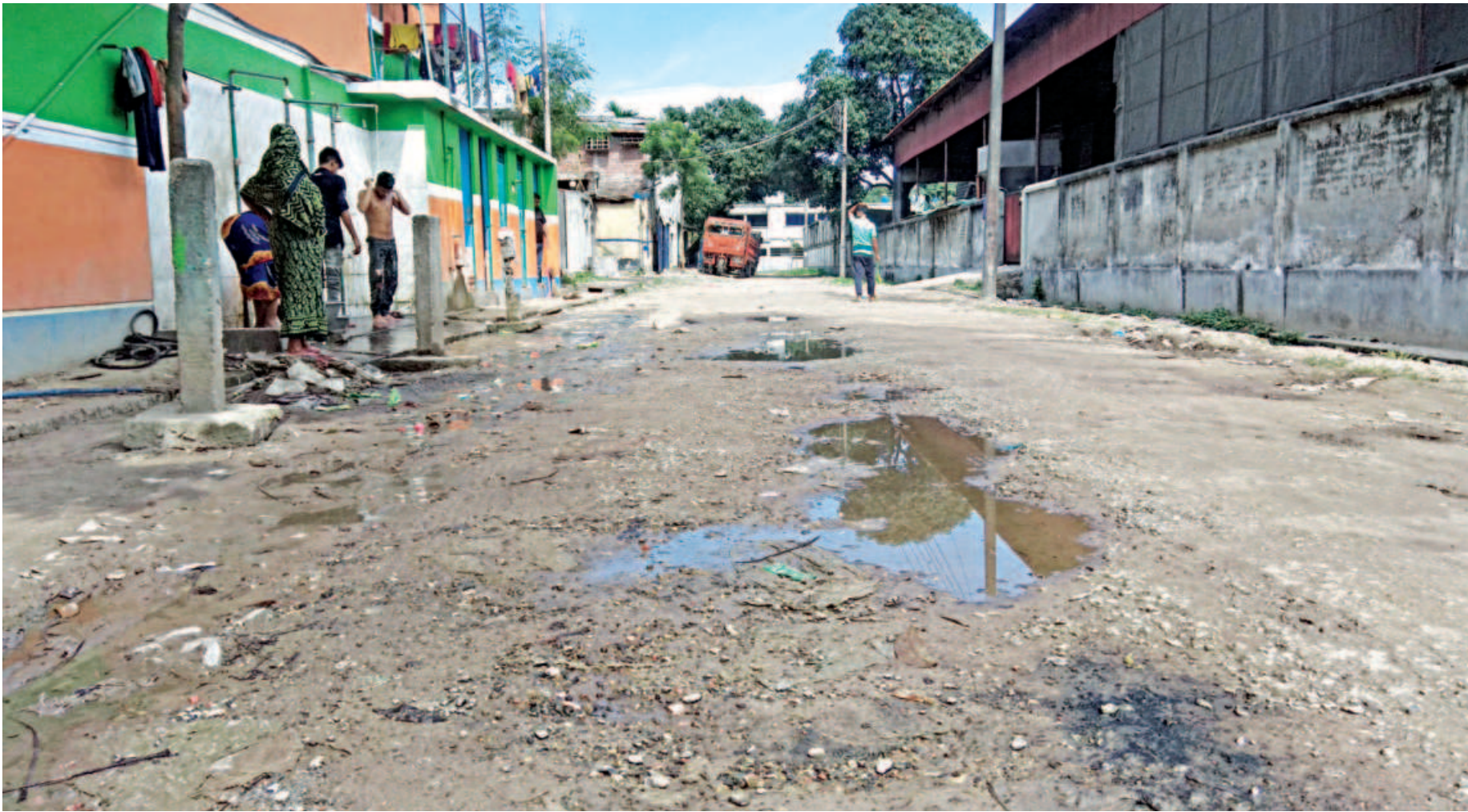
Coupled with a poor drainage system, these dilapidated roads at the BSCIC industrial estate in Chapainawabganj become flooded during the rainy season and hamper business activities.
