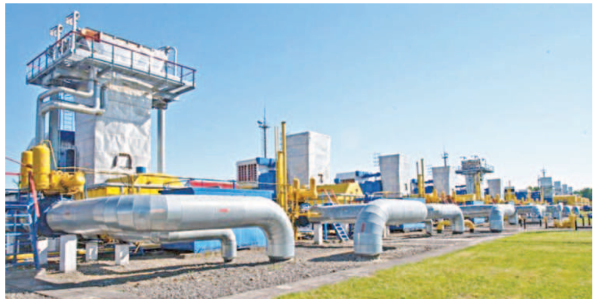
A view of pipelines at the Bilche-Volytsko-Uherske underground gas storage facility, the largest in Europe, in the Lviv region of western Ukraine.
