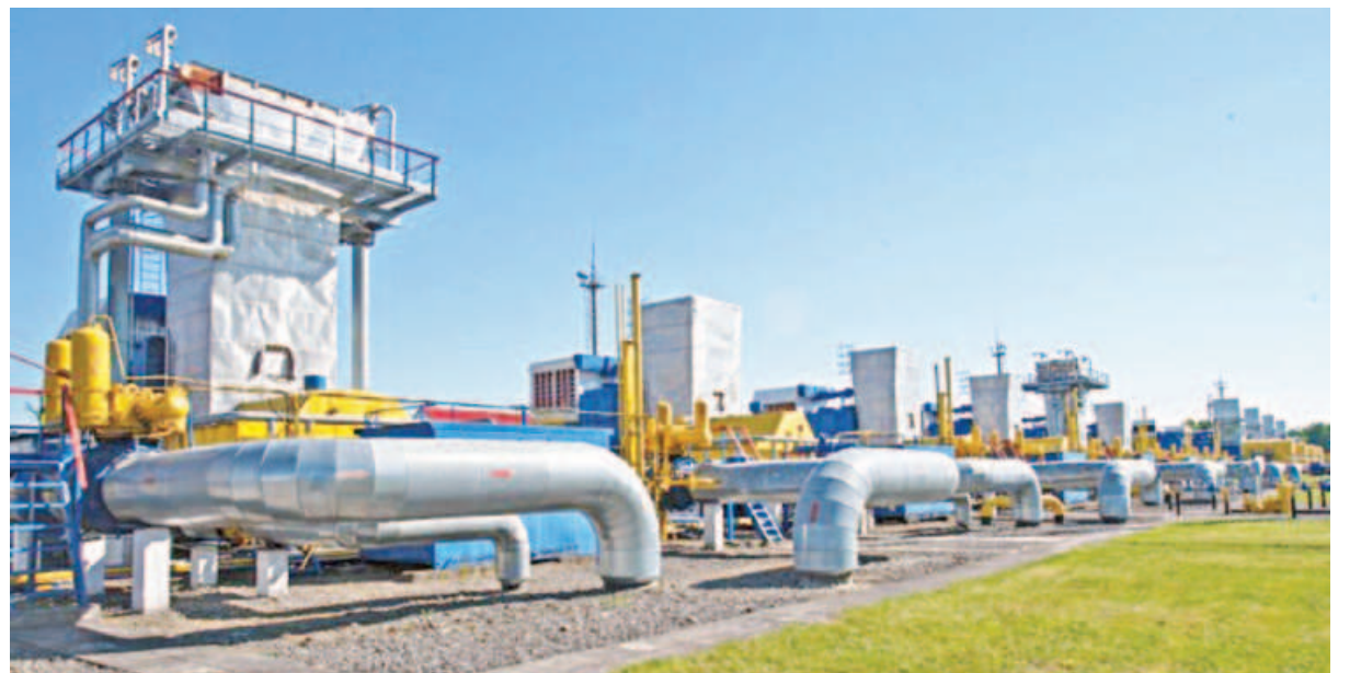
A view of pipelines at the Bilche-Volytsko-Uherske underground gas storage facility, the largest in Europe, in the Lviv region of western Ukraine.
