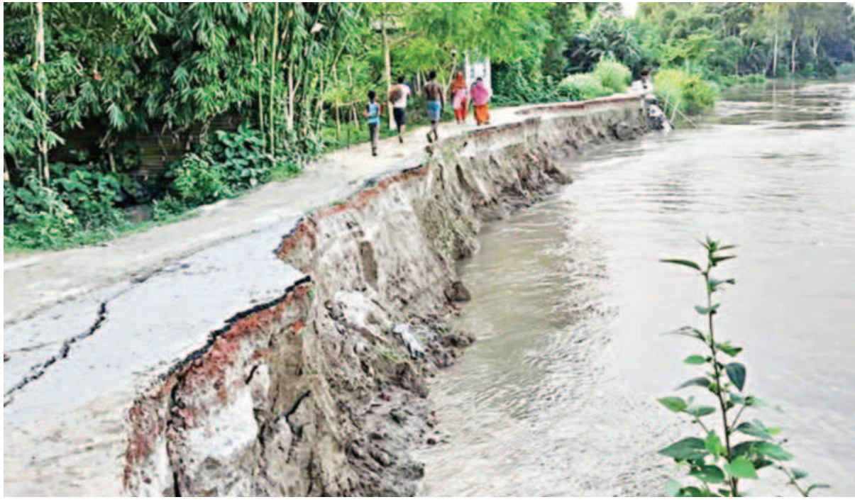
Large portion of this paved road under Kanchanpur union in Tangail's Basail upazila has been devoured by the Jhenai river a few days ago. PHOTO: STAR
