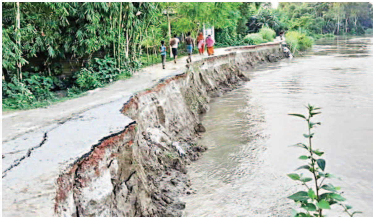
Large portion of this paved road under Kanchanpur union in Tangail's Basail upazila has been devoured by the Jhenai river a few days ago.
