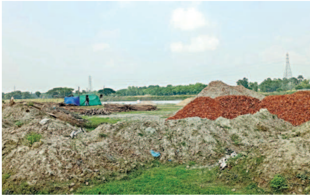
Construction materials, including bricks, concrete and sand, are kept right on the bank of Old Brahmaputra river, further endangering the waterbody, which has already been suffering due to pollution and encroachment. This photo was taken recently. PHOTO: STAR
