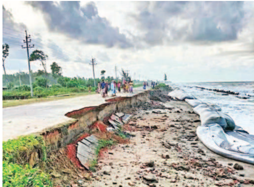
A part of Cox's Bazar-Teknaf Marine Drive damaged by Cyclone Sitrang. PHOTO: MOHAMMAD ALI JINNAT
