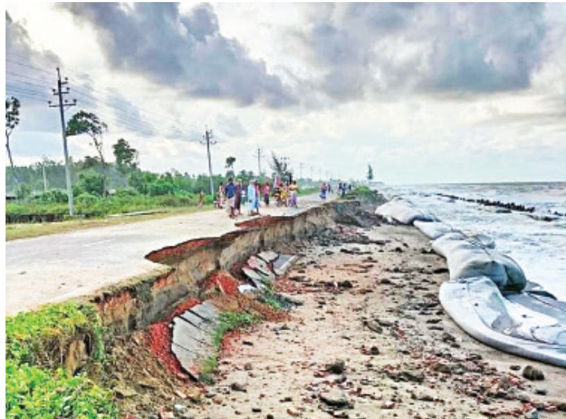
A part of Cox's Bazar-Teknaf Marine Drive damaged by Cyclone Sitrang. PHOTO: MOHAMMAD ALI JINNAT
