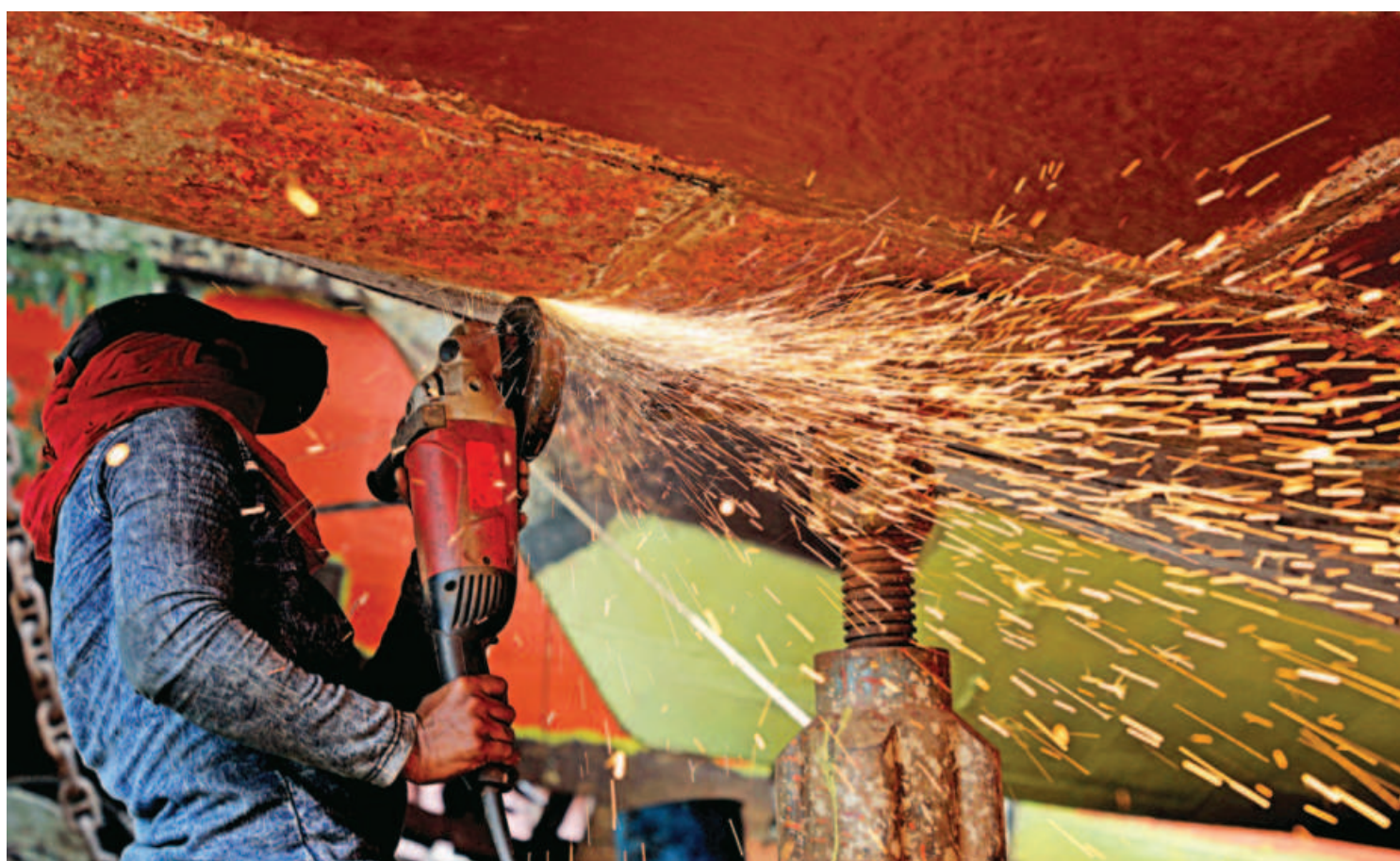
With barely any safety gear on, a worker grinding a metal plate while repairing a launch in Dhaka's Keraniganj dockyard. Most workers in such places have to work in precarious conditions, as the authorities concerned turn a blind eye to the safety of their employees. The photo was taken recently.
