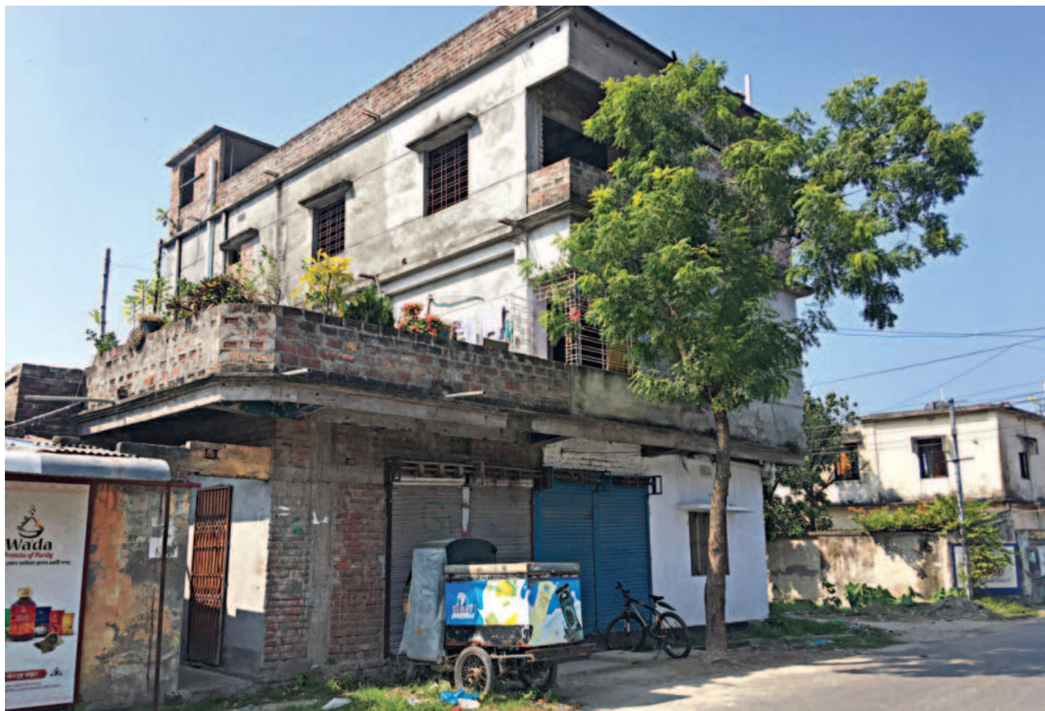
The Keramat Rice Mills situated on two plots inside the BSCIC industrial estate in Rajshahi seems more like a ramshackle apartment complex than an industrial unit as its owners have long been renting it out as such. Following repeated warnings from the estate authorities, the residents have set up small-scale light engineering units to allay concerns.
