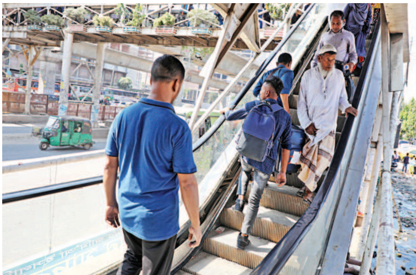
Even though there is an escalator for the footbridge near the Hazrat Shahjalal International Airport, people have to climb the stairs as it is broken. The photo was taken yesterday.
