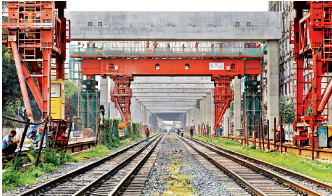
A section of the under-construction Dhaka Elevated Expressway near the capital's Chairmanbari area. Construction for the expressway means that much of the work for the Dhaka-Tongi-Joydebpur rail expansion project is halted. The expressway is being constructed over the rail tracks from Kawla to Kamalapur, which forms a major part of the area of the rail expansion project.
