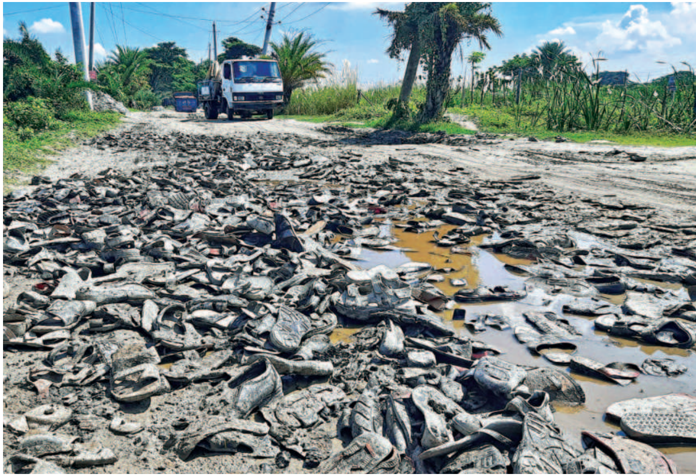
As the authorities do not repair the pothole-riddled Abu Naser Bypass Road in Khulna city, despite the sufferings of a few hundred families there, locals try to fill the holes with worn-out shoes. The photo was taken yesterday.
