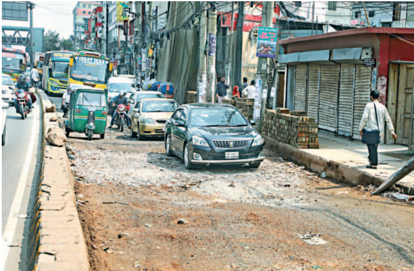
The road under the Jatrabari flyover in the capital's Shonir Akhra area remains damaged for over three months, but the authorities seem to be uninterested in fixing it. Locals say accidents take place frequently here on the rainy days. Long tailbacks have become a regular scene here. The photo was taken recently.
