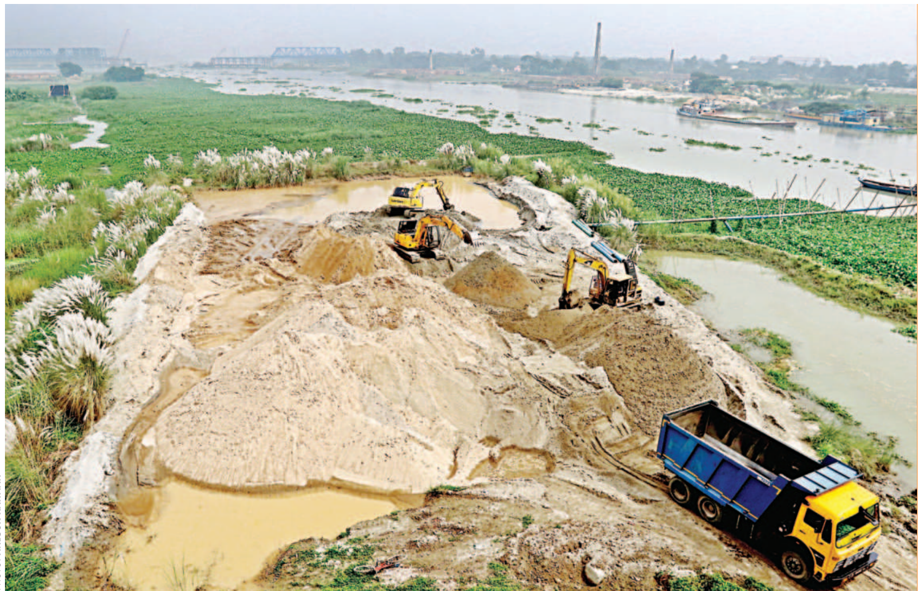
Excavators lifting sand piled up on the bank of the Dhaleshwari river in Munshiganj's Sirajdikhan upazila yesterday. The sand will be loaded onto trucks and taken away for construction work. Ships carry the sand from various regions and deposit it on the bank, resulting in this portion of the river becoming narrower over the years.
