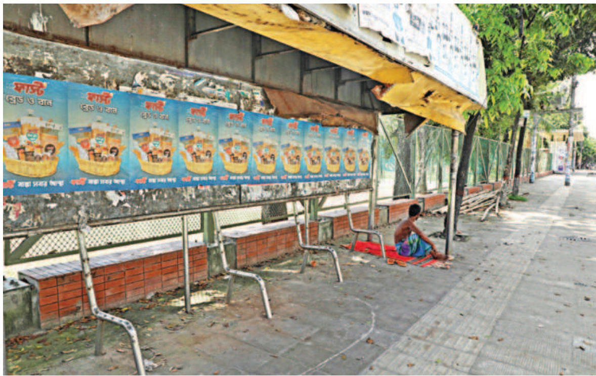
A bus stop has the rod beams in place for benches to be set, but the seating arrangement is conspicuously absent, compelling waiting passengers to either stand. The photo was taken from the capital's Kalabagan area yesterday. PHOTO: AMRAN HOSSAIN
