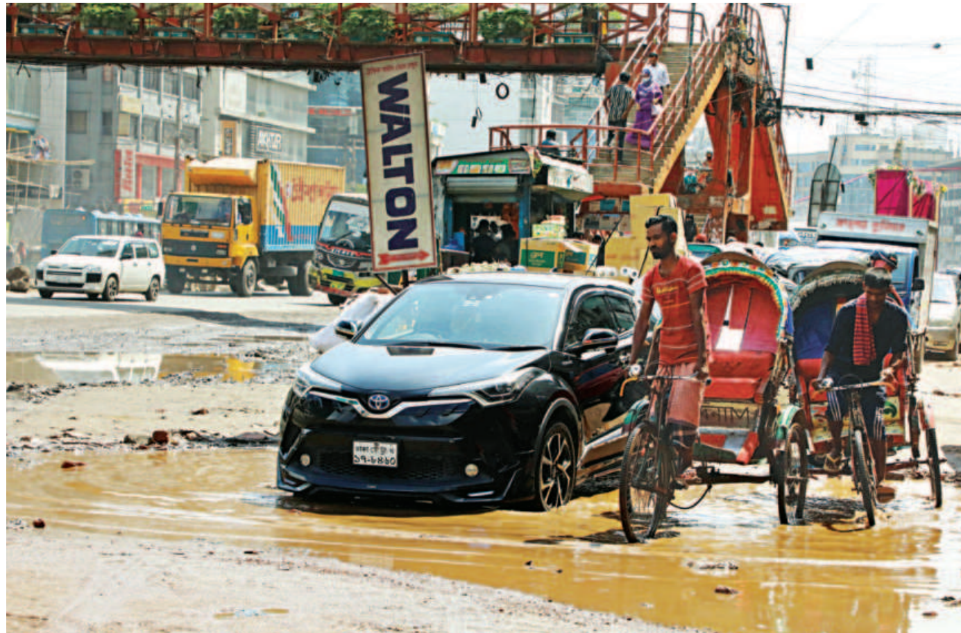
Massive potholes causing frequent traffic gridlocks and damaging vehicles in the capital's Uttara. According to locals, this pothole was detected around two months ago, but the authorities never paid any heed to repair it. The photo was taken near Rajlakkhi Complex yesterday.
