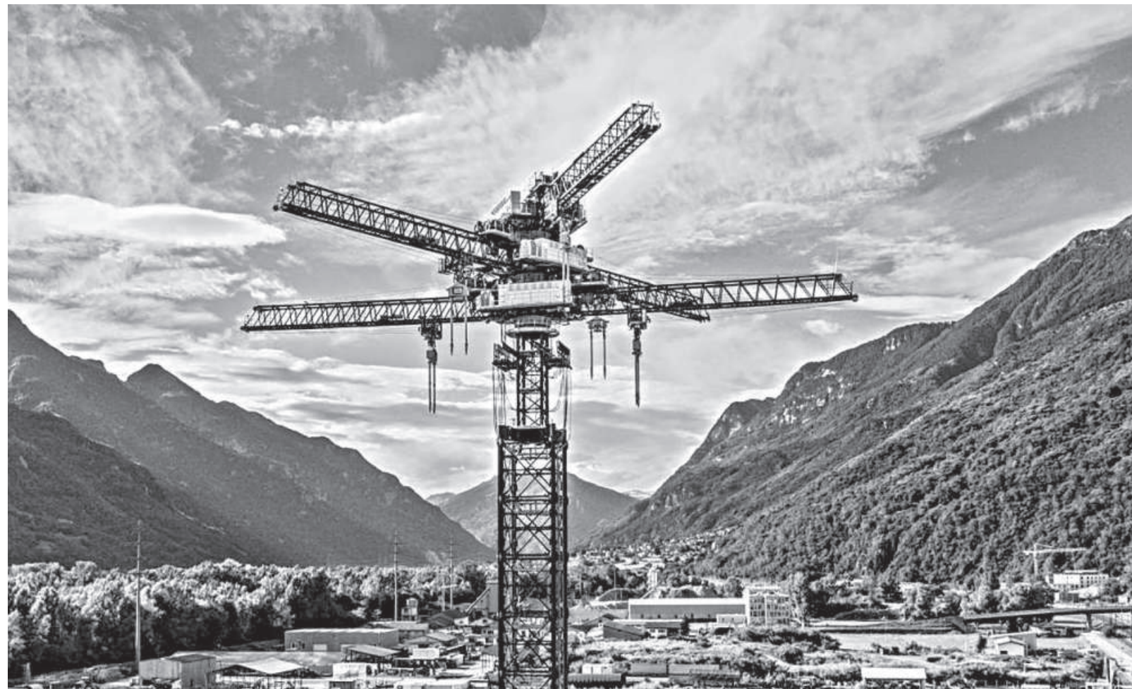
SOURCE: ENERGY VAULT
