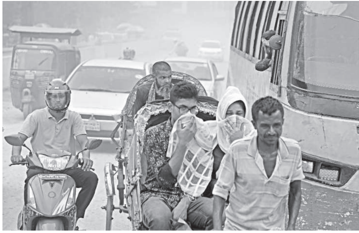
Even with the rainfall over the last few days, dust engulfed the Agargaon area, owing to the development work of a mega project. Commuters were seen covering their faces and squinting their eyes while using the road yesterday.
