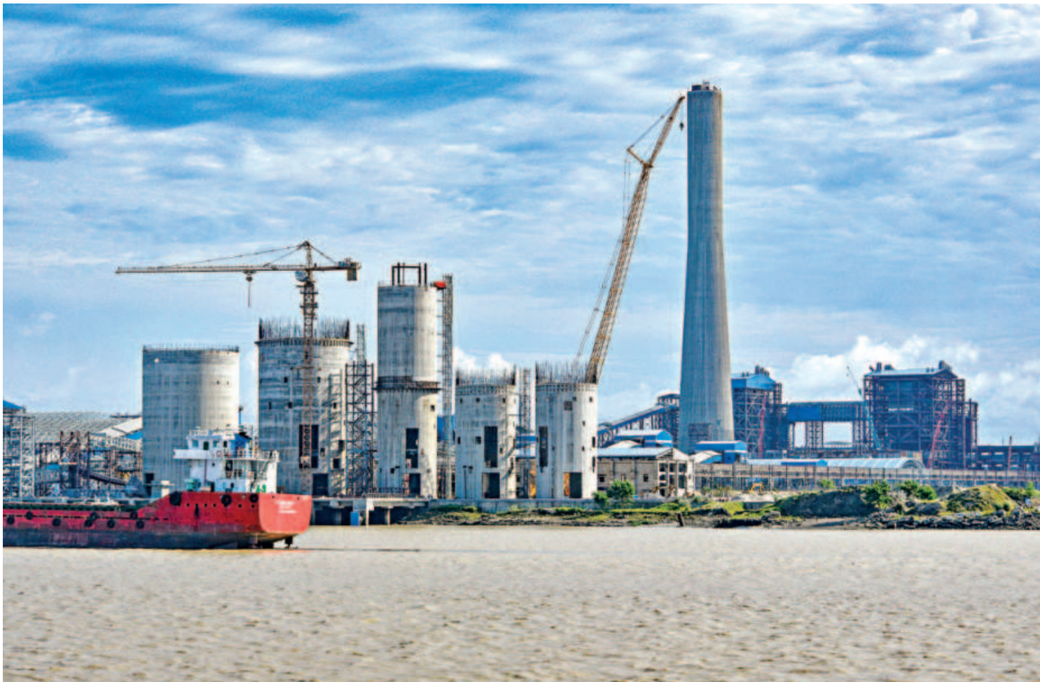
The 1,320MW Maitree super thermal power project at Rampal in Bagerhat district, 14 kilometres north-east of the Mongla port and 14 kilometres north-west of the Sundarbans mangrove forest. It is costing about $2 billion, of which $1.6 billion is being sourced as Indian Development Assistance under a concessional financing scheme. The photo was taken recently.
