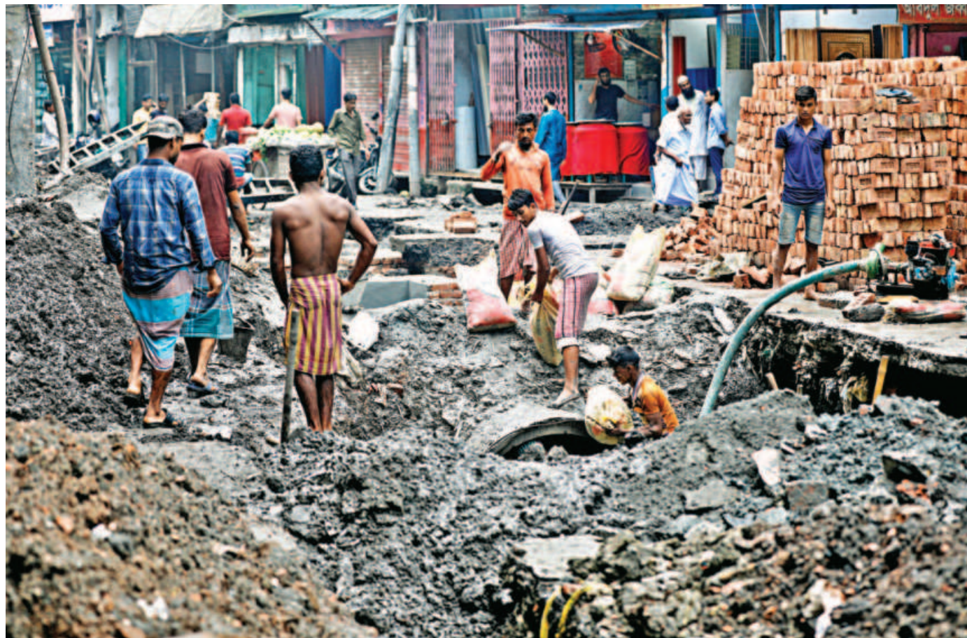
French Road in Naya Bazar area of the capital has been dug up entirely to install large sewerage pipes. Dhaka South City Corporation started the project around six months ago, apparently without considering how the work would affect locals. The photo was taken yesterday.
