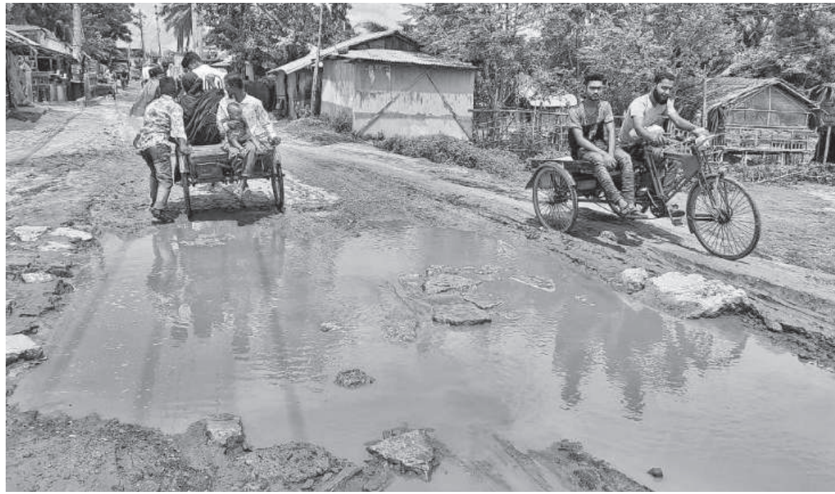
For almost eight years now, commuters have been crossing the Bir Srestha Ruhul Amin Road in Rupsha upazila of Khulna with great difficulty. Often times, rickshaw and van pullers have to get down and drag their vehicles on the muddy road amid numerous potholes.
