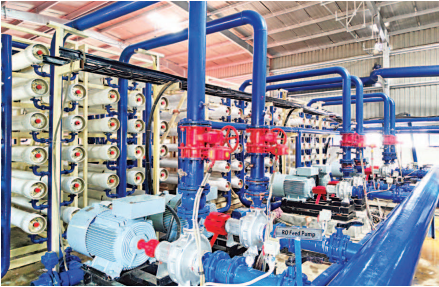
A water treatment plant set up near the Patenga silo jetty in Chattogram, having a capacity to purify three million gallons of water of the Karnaphuli river daily. Constructed by Dhaka-based Sigma Group, the facility was inaugurated yesterday to meet a shortage of water at 148 factories in Chattogram Export Processing Zone.
