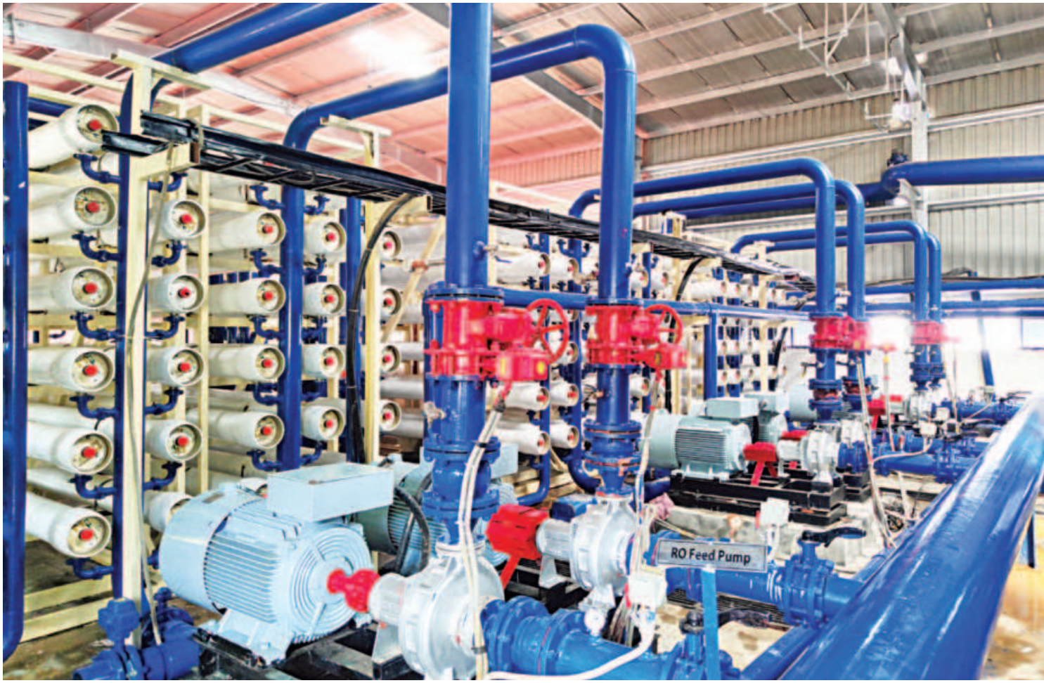
A water treatment plant set up near the Patenga silo jetty in Chattogram, having a capacity to purify three million gallons of water of the Karnaphuli river daily. Constructed by Dhaka-based Sigma Group, the facility was inaugurated yesterday to meet a shortage of water at 148 factories in Chattogram Export Processing Zone.
