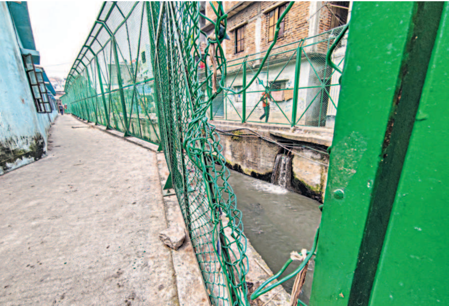
Locals removed parts of an iron fence, set up by DSCC to prevent people from dumping household wastes into Hazaribagh canal. Although authorities often face the music regarding environment pollution, it's about time the residents hold up their end of the bargain in saving rivers and canals around them. This photo was taken at Hazaribagh area recently.
