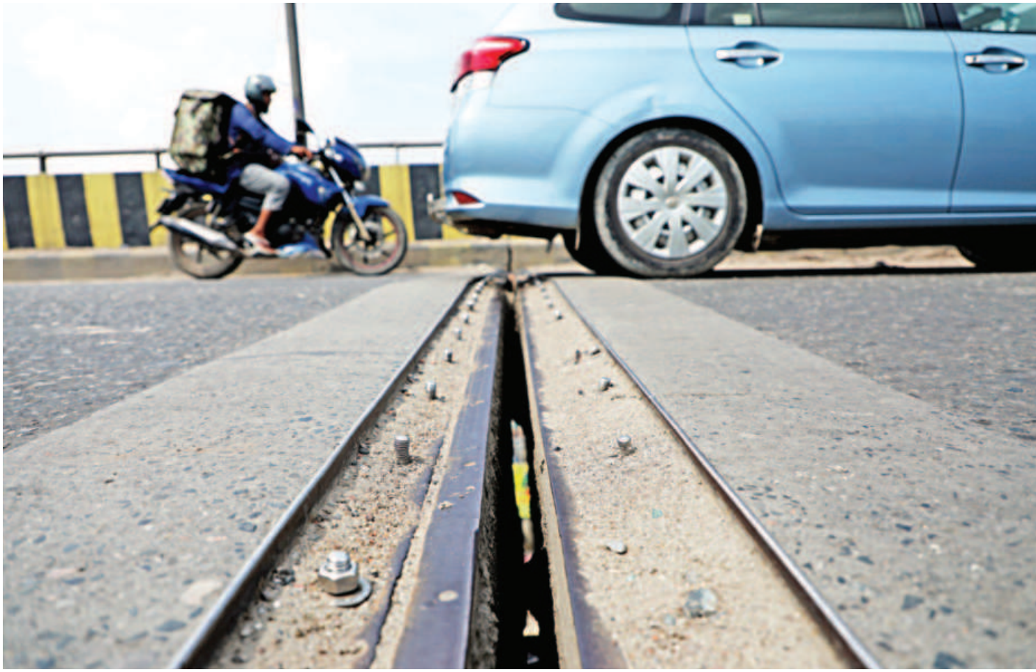
Gaps are usually placed at the junctions of bridges to ensure that damage doesn't occur, as bridges expand and contract due to vibrations. This section again is wrapped with rubber to ensure that vehicles can run smoothly. However, the rubber on the expansion joint of Demra's Sultana Kamal Bridge has completely come off. The rubber on other parts of the bridge has also eroded, signing caution to the authorities concerned to fix them, before it hampers the bridge's overall structural integrity. This photo was taken yesterday.
