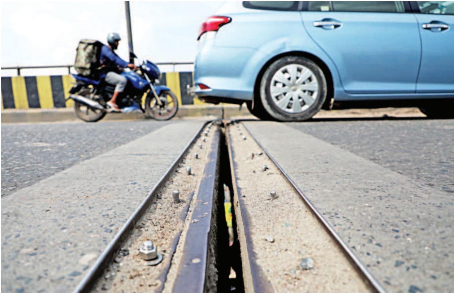
Gaps are usually placed at the junctions of bridges to ensure that damage doesn't occur, as bridges expand and contract due to vibrations. This section again is wrapped with rubber to ensure that vehicles can run smoothly. However, the rubber on the expansion joint of Demra's Sultana Kamal Bridge has completely come off. The rubber on other parts of the bridge has also eroded, signing caution to the authorities concerned to fix them, before it hampers the bridge's overall structural integrity. This photo was taken yesterday. PHOTO: PALASH KHAN
