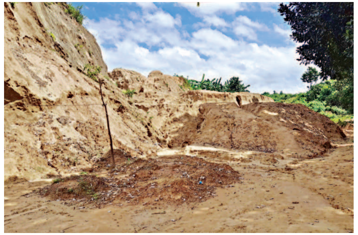
A hill being cut to build houses at Uttar Baluchar Jonaki in Sylhet city. Local law enforcers seem to turn a blind eye to this utter disregard for environment laws. The photo was taken recently.
