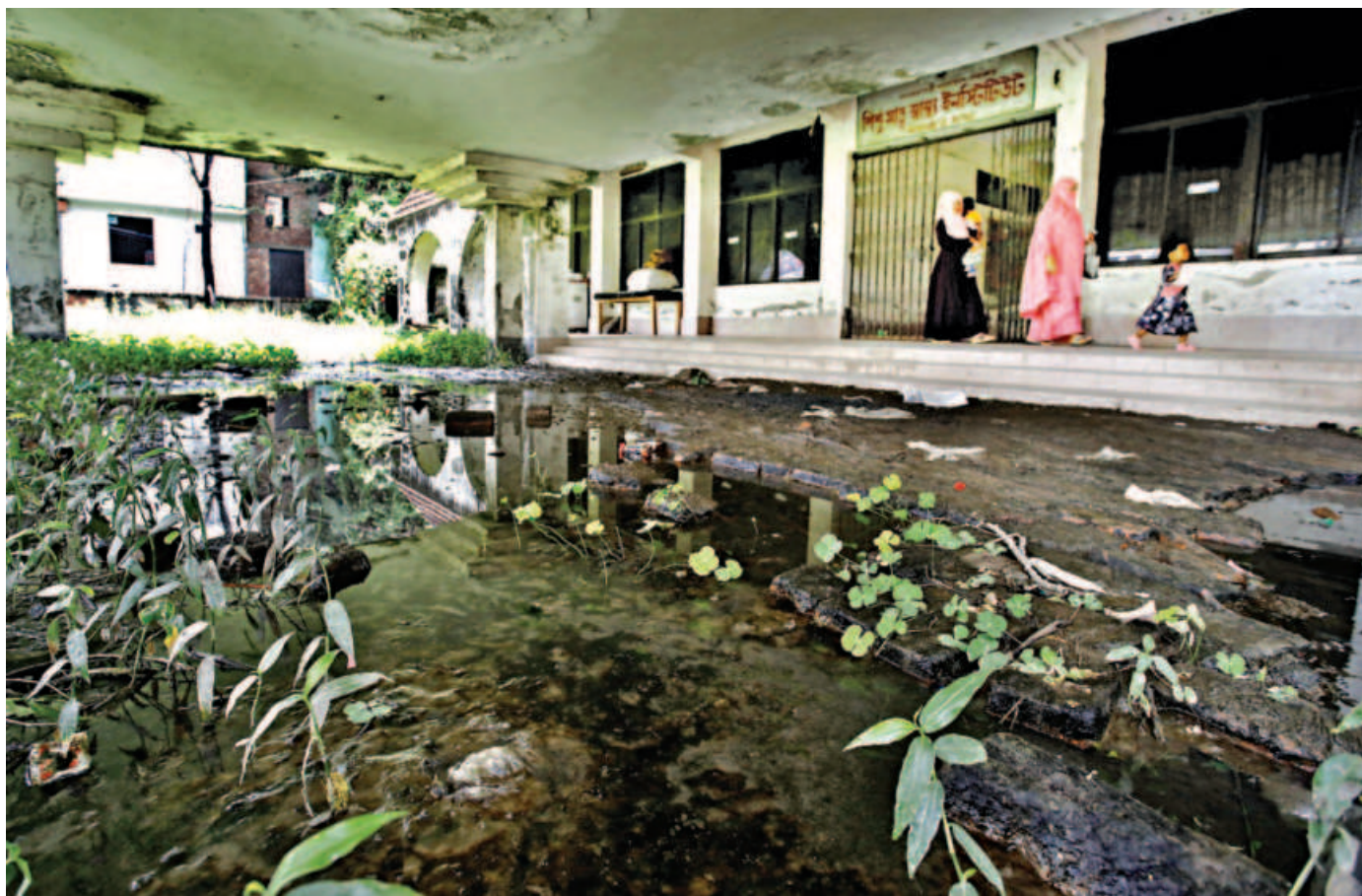
The entrance to the Jalkuri branch of the Institute of Child and Mother Health in Narayanganj is waterlogged, with weeds springing up from the soil. This place has become a perfect breeding ground for mosquitoes, thanks to poor drainage. This is causing unnecessary suffering for patients. The photo was taken yesterday.
