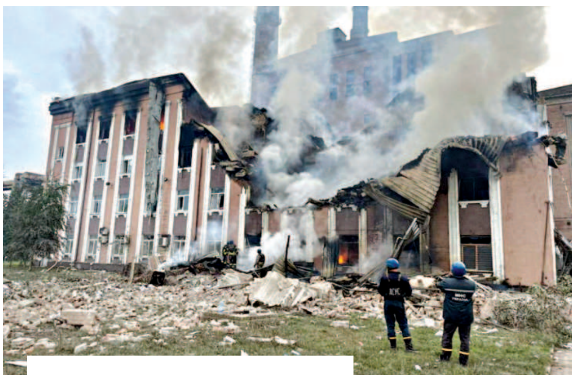
A part of the Sloviansk Thermal Power Plant damaged by a Russian military strike in the village of Mykolaivka, Donetsk region, Ukraine. Inset, A woman meets her friends on a street as she returns to her liberated home village after six months and eleven days in Troitske, Kharkiv. Both photos were taken on Sunday.
