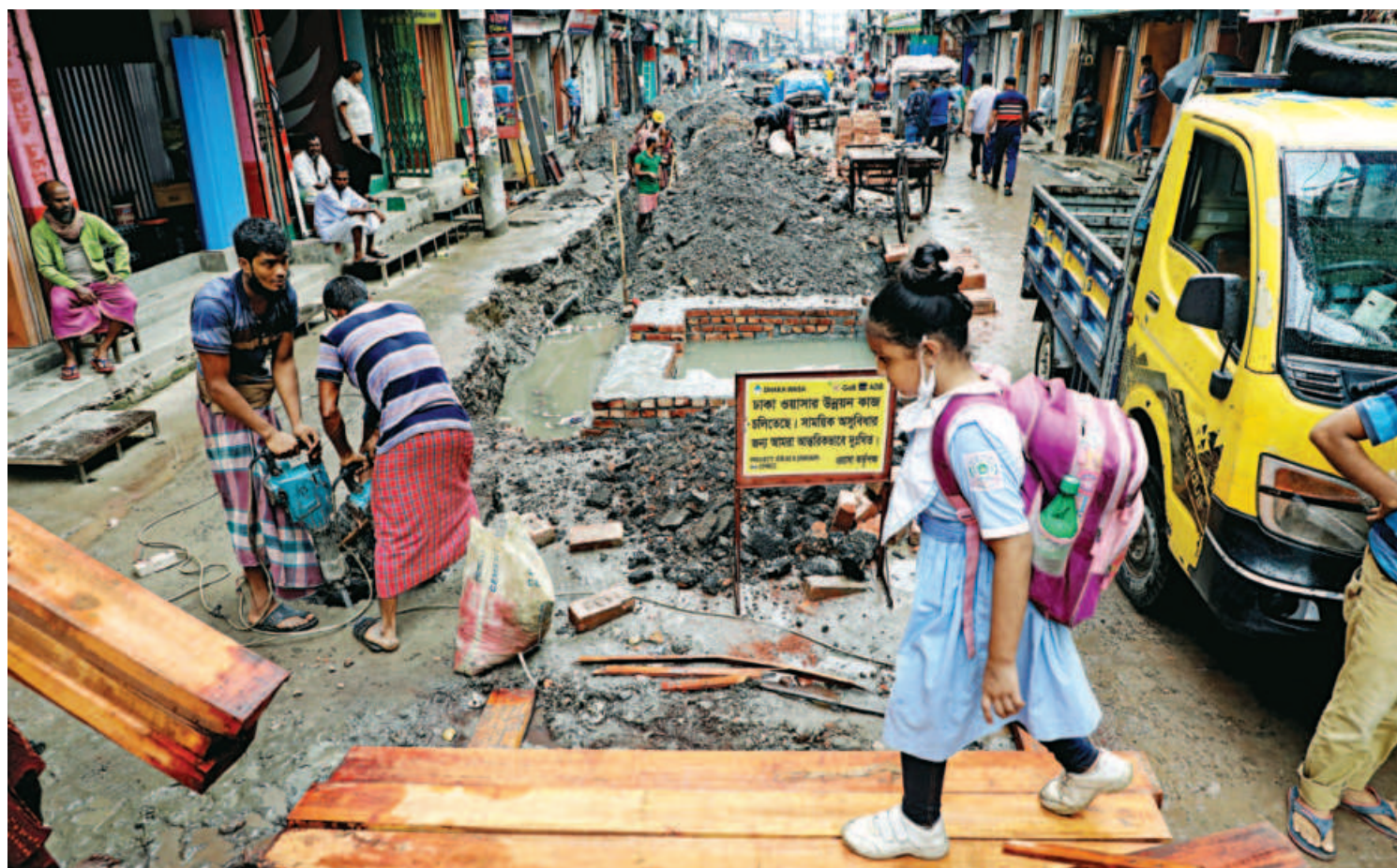
A girl walks over a wooden plank used for covering a manhole on the busy Naya Bazar road in Old Dhaka yesterday. As part of an ongoing city development work of Wasa, the road has been dug up and left like this for a while now without ensuring any safety measures. As a result, commuters have to face great difficulties to use the road.
