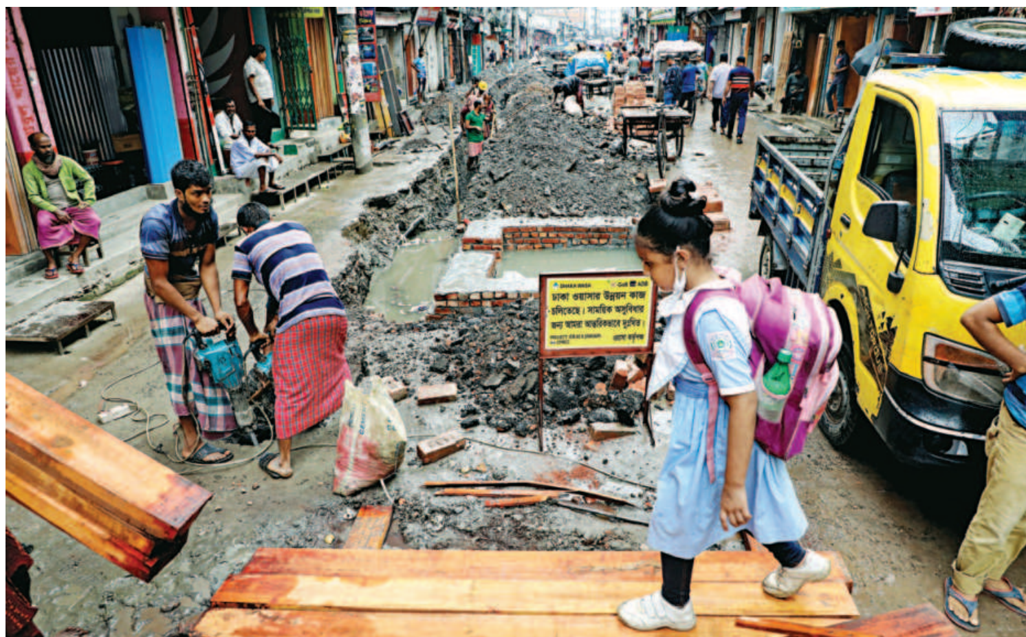
A girl walks over a wooden plank used for covering a manhole on the busy Naya Bazar road in Old Dhaka yesterday. As part of an ongoing city development work of Wasa, the road has been dug up and left like this for a while now without ensuring any safety measures. As a result, commuters have to face great difficulties to use the road.
