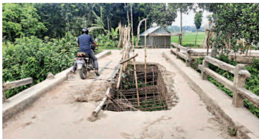
Part of the deck of this bridge on Alamdanga Canal in Jhenidah's Shailakupa upazila remains unrepaired for years, making it difficult for vehicles to cross it.
