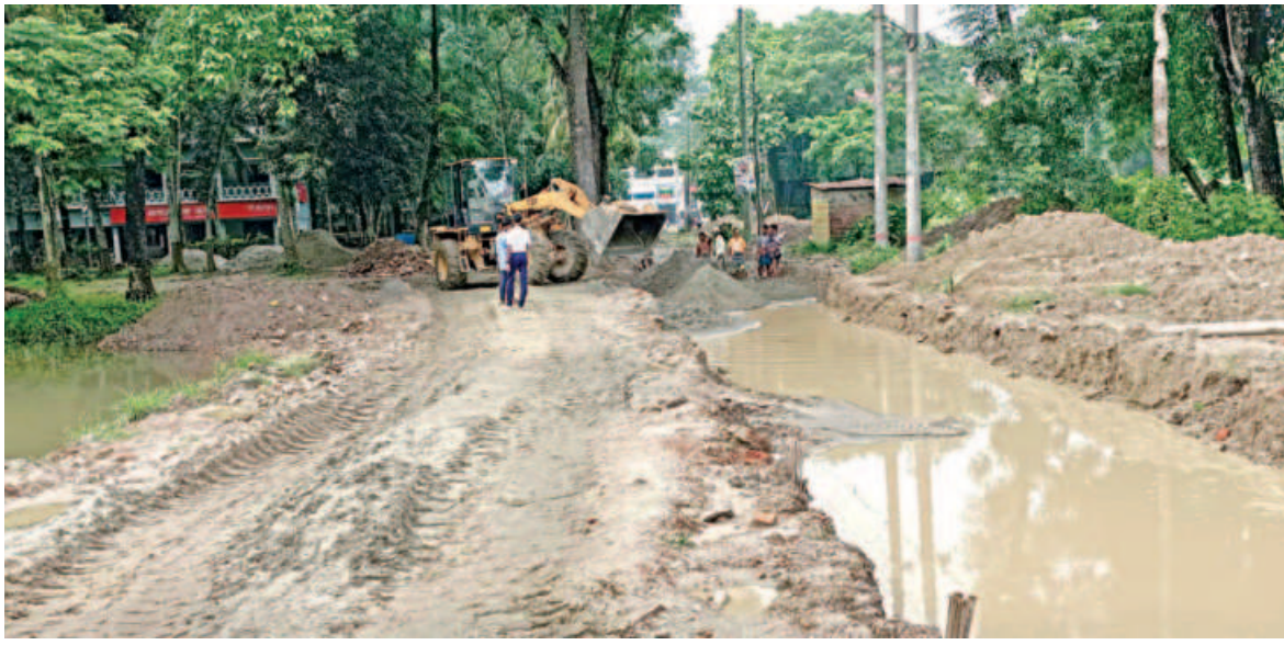
The ongoing work for a drain pipe in Mymensingh city is causing immense sufferings for commuters. With SSC exams nearing, students of nearby schools may face great difficulty to reach exam halls. PHOTO: STAR
