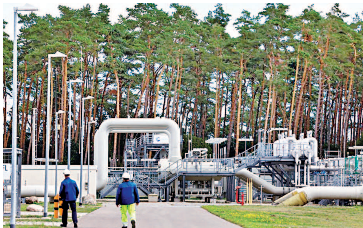
The Nord Stream 1 Baltic Sea pipeline and the transfer station of the Baltic Sea Pipeline Link in the industrial area of Lubmin in Germany. G7 members have already limited or suspended their Russian petroleum purchases, but for the plan to be effective, other countries like India and China, some of Russia's most important clients, have to join the fray.
