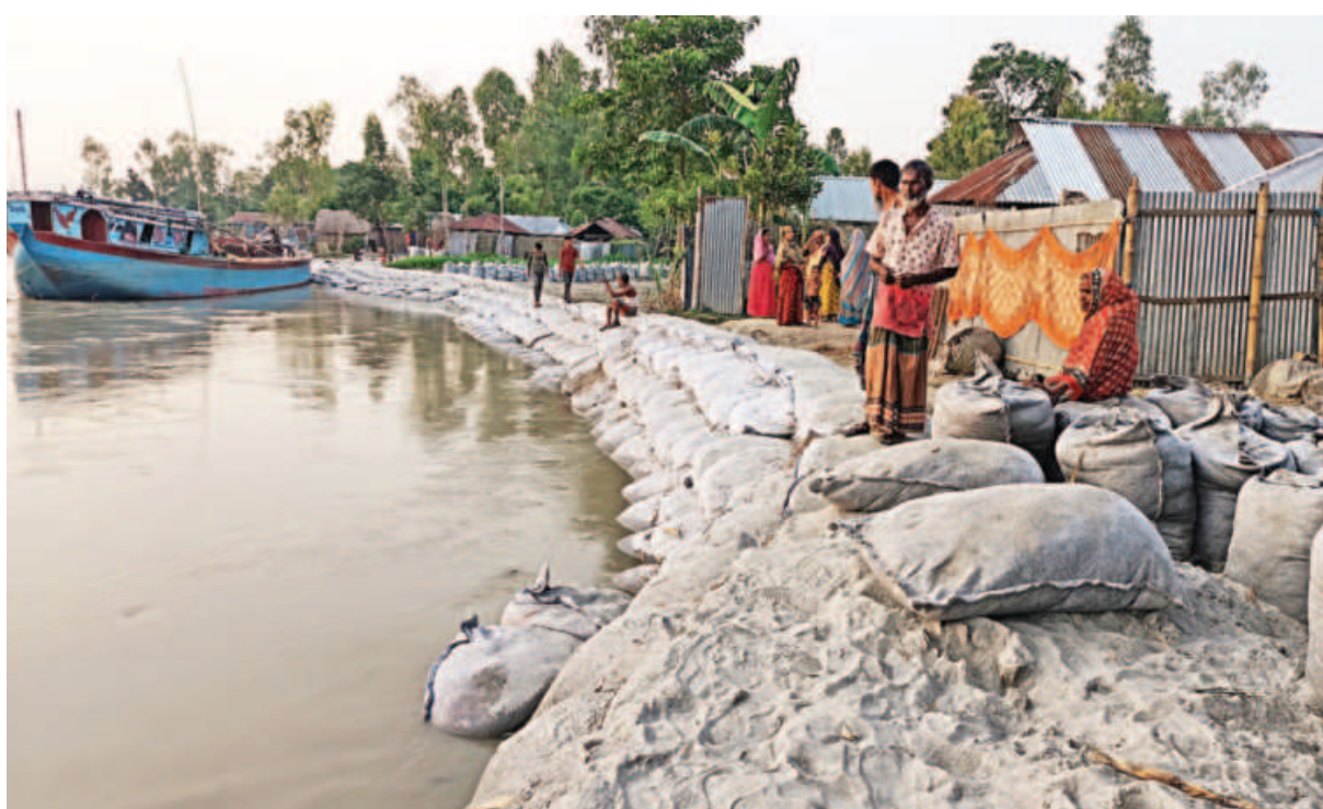
WDB dumping sand bags in different erosion-hit areas to protect the river banks. The photo was taken from Purbo Kalmati village in Lalmonirhat Sadar upazila.
