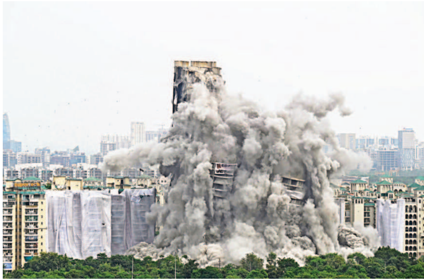
A controlled implosion demolishes the 100-metre-high residential "Twin Towers" in Noida on the outskirts of New Delhi, yesterday. Two illegally built residential high-rises were demolished near India's capital in a rare crackdown on developers who cut corners and swindle unsuspecting home-buyers. PHOTO: AFP
