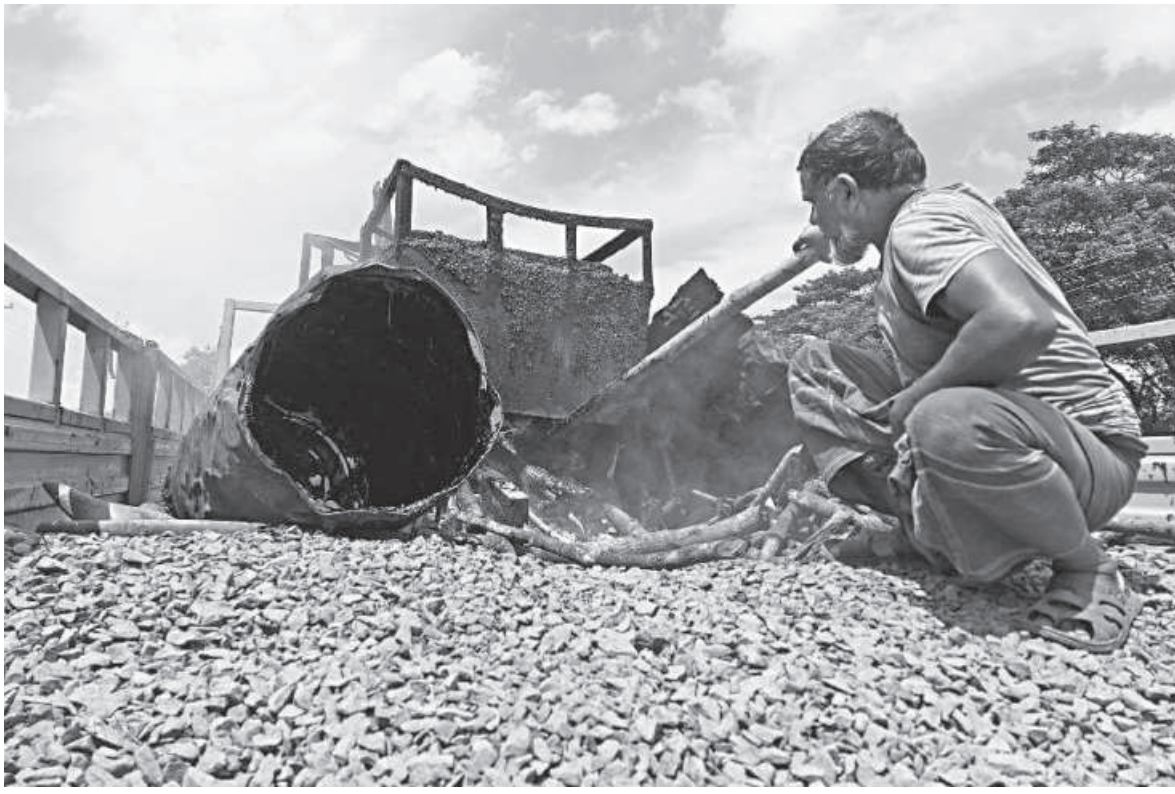
A worker melting pitch in a boiler machine for emergency repairs of potholes on Barishal-Dhaka highway. This photo was taken in Rahmatpur area of Barishal's Babuganj upazila.
